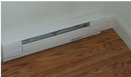
Electric Baseboard Heat
