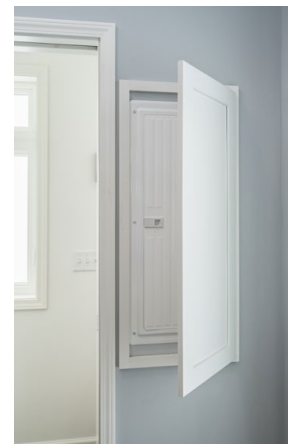
Cabinet Door Over Panel Box
